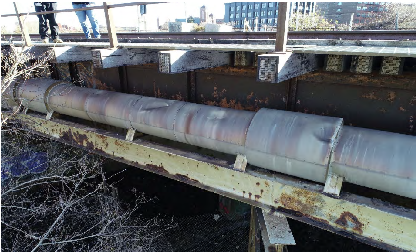
Denting along pipe jacketing near eastern end, looking south east
